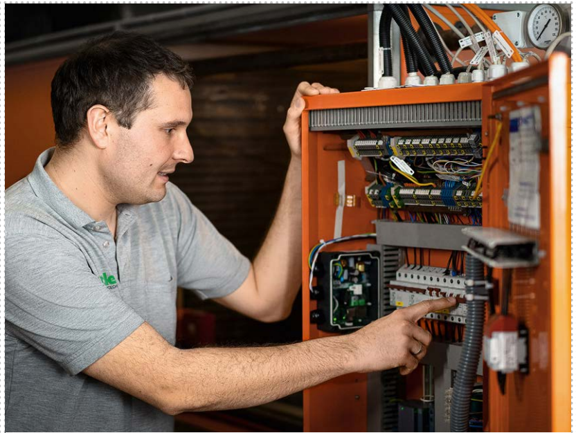
FIGURE 2: The system's control cabinet was still well maintained and could therefore be supplemented with sensors and ebm-papst neo gateway without great effort.
